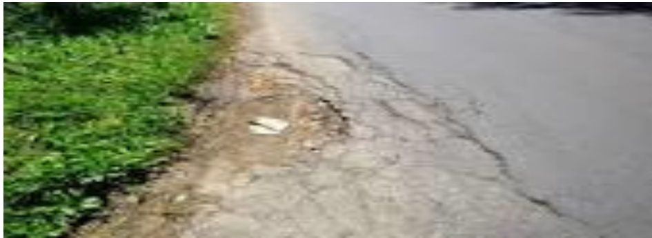
Gambar 3.6 Retak Pinggir (Shahin, 2005)
