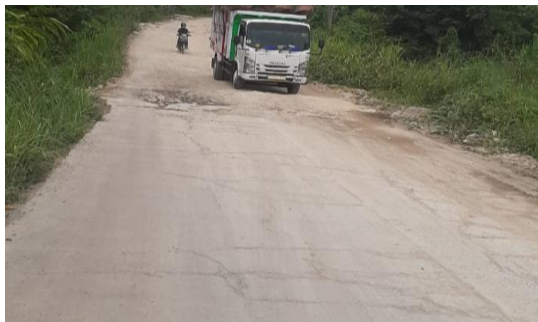
Gambar 2.1 Retak halus ( hair cracking )
