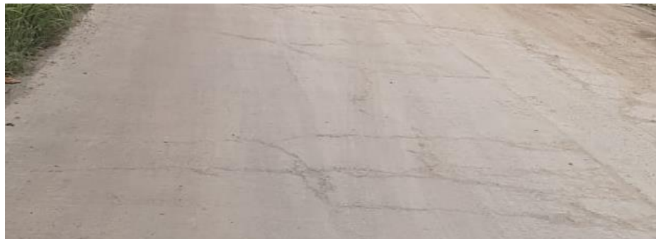
Gambar 2.1 Retak halus ( hair cracking )
