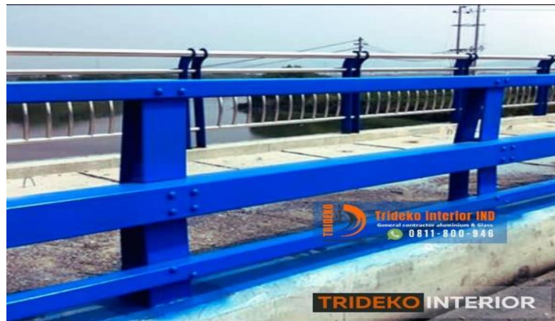
Gambar 2.5 Pagar pengaman (Guard Railing)
